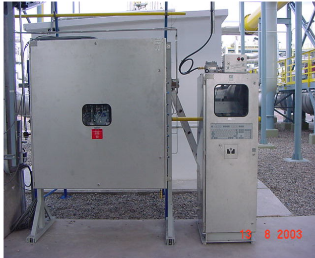
Figure 2 Typical Installation - the Sampling System and Analyser in Purged Cabinet
